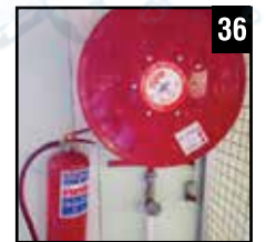
Fire Hydrant & Hose Reels
